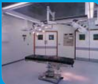
Operating Theatre - Laminar Flow Canopy
