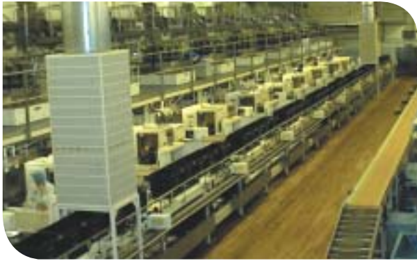
KP - Displacement Air Conditioning
