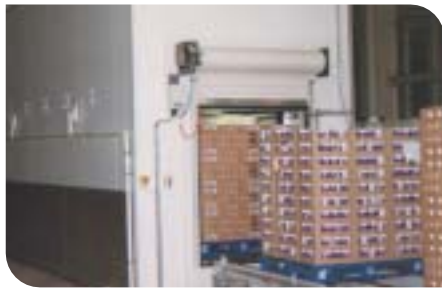
Muller Dairy - Cooling Tunnel
