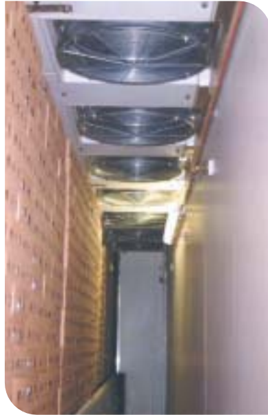
Muller Dairy - Cooling Tunnel
