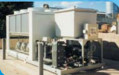
Stonegate Foods - Process Chiller
