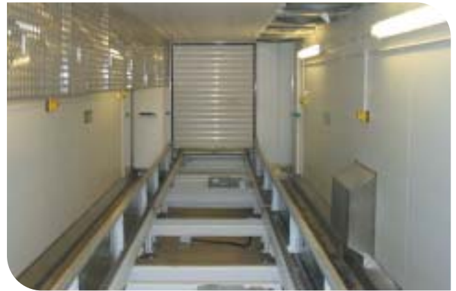
Muller Dairy - Cooling Tunnel
