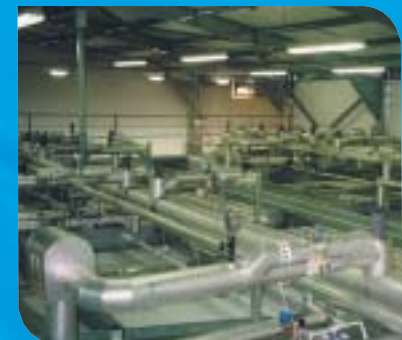
Uniq Foods - Ammonia Refrigeration Pipework
