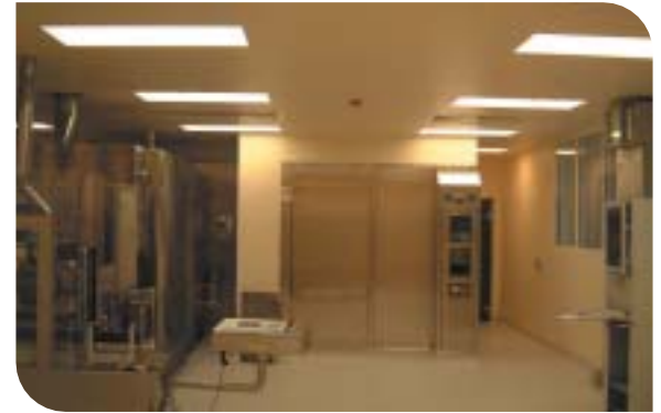
Patheon - Clean Room
