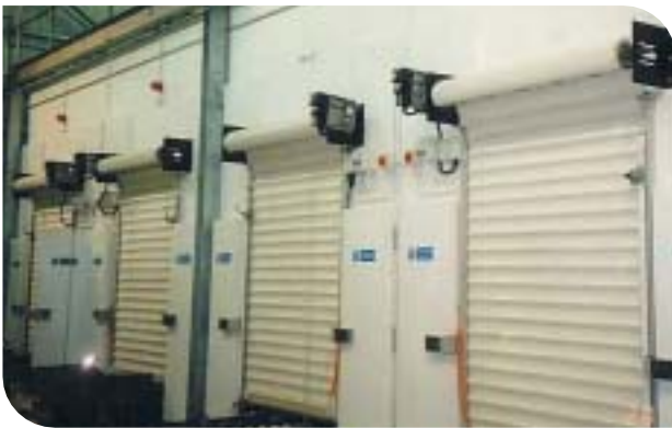
Uniq Foods - Multi Lane Cooling Tunnels
