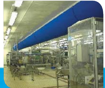
Dairy Crest - High Care Air Conditioning
