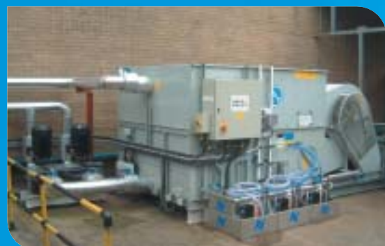
Nestlé - Cooling Tower, Cuddington
